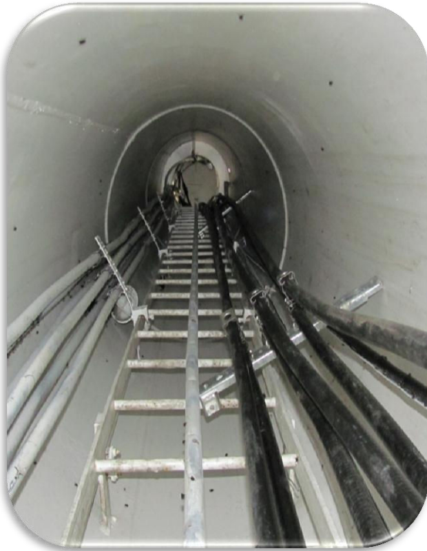
Photo 1 (a cellular company has installed cables on the side and face of ladder)
